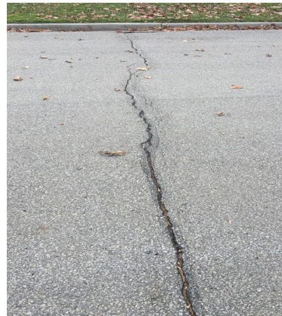
Example of crack identified > 5 cm
